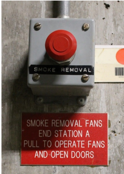
Figure 2. Smoke Removal Button
