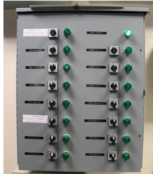
Figure 3. Fan Controls in the MCC
